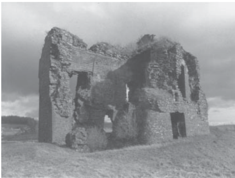
Fig. 4 Torthorwald Castle from N.W., prior to collapse of N.E. corner in 1993.
