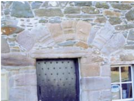
Figure 5 Wall Hill, Netherlaw sandstone carved stone arch mouldings, probably from Dundrennan, re-used in the Tolbooth, Kirkcudbright
