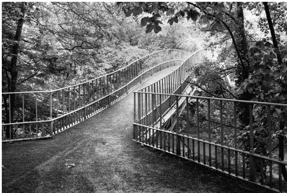
Figure 2. Duchess Bridge, Langholm in 1984, view from the south showing the outward splay of the handrails. (Copyright RCAHMS SC 361838)
